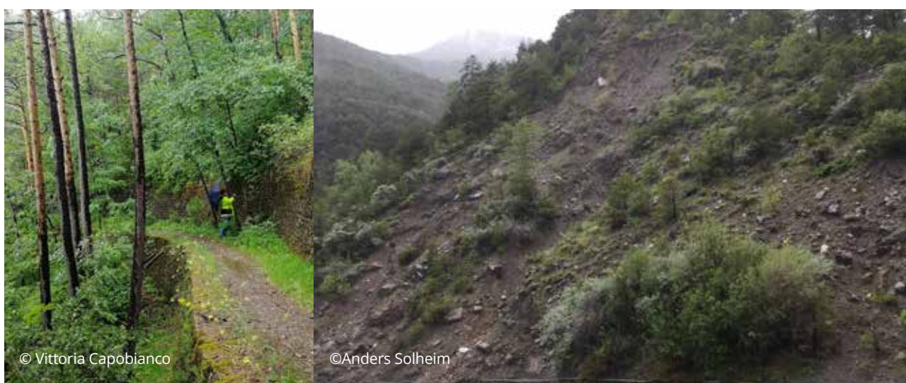
Image 4.3 A vegetated and terraced wall on the slopes of Biescas (Spain) today, the result of implementing a nature-based solution more than 100 years ago (left), and a till slope in Santa Elena (Spain) with frequent rockfall problems (right). It will be terraced, drained and revegetated, inspired by the traditional approach taken at Biescas
